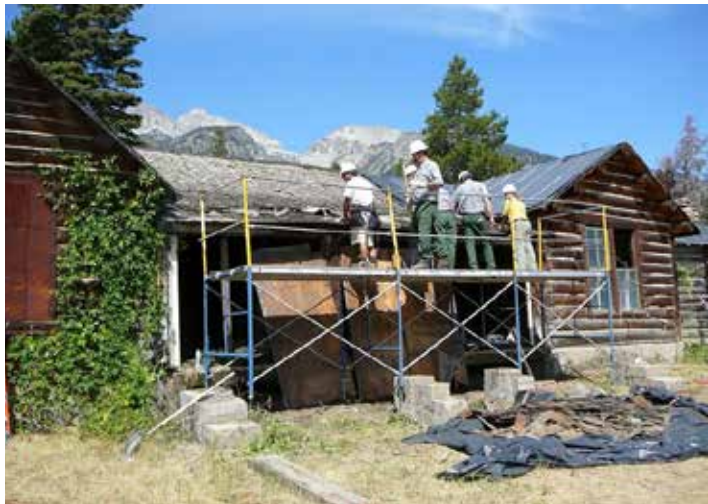
Historic preservationists restore White Grass Ranch at Grand Teton National Park. NPS /Grand Teton NP photo
