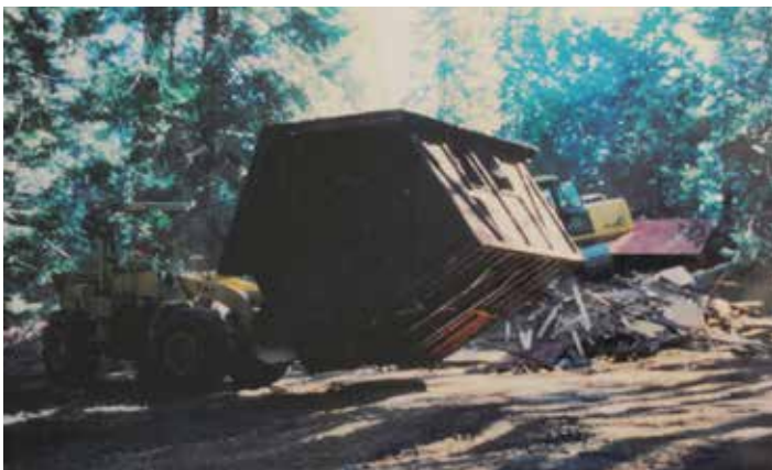
Loaders and excavators remove entire buildings in the Giant Forest during a reclamation period from 1997 to 1999. NPS photo
